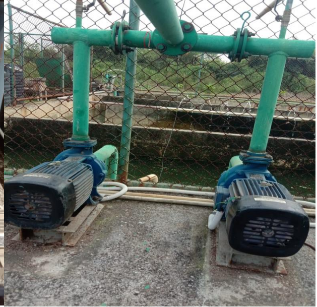
Filter Feed Pump
