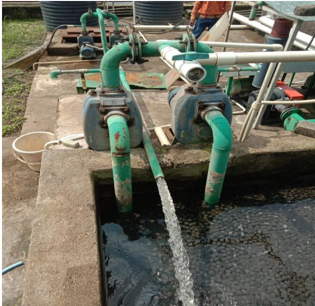
Bio Tower Airson Pump
